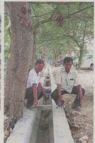
Residents Ping (left) and Maniam showing one of the tree stumps in the way of the newly constructed drain. They worry the roots from the tree could damage the drains.
